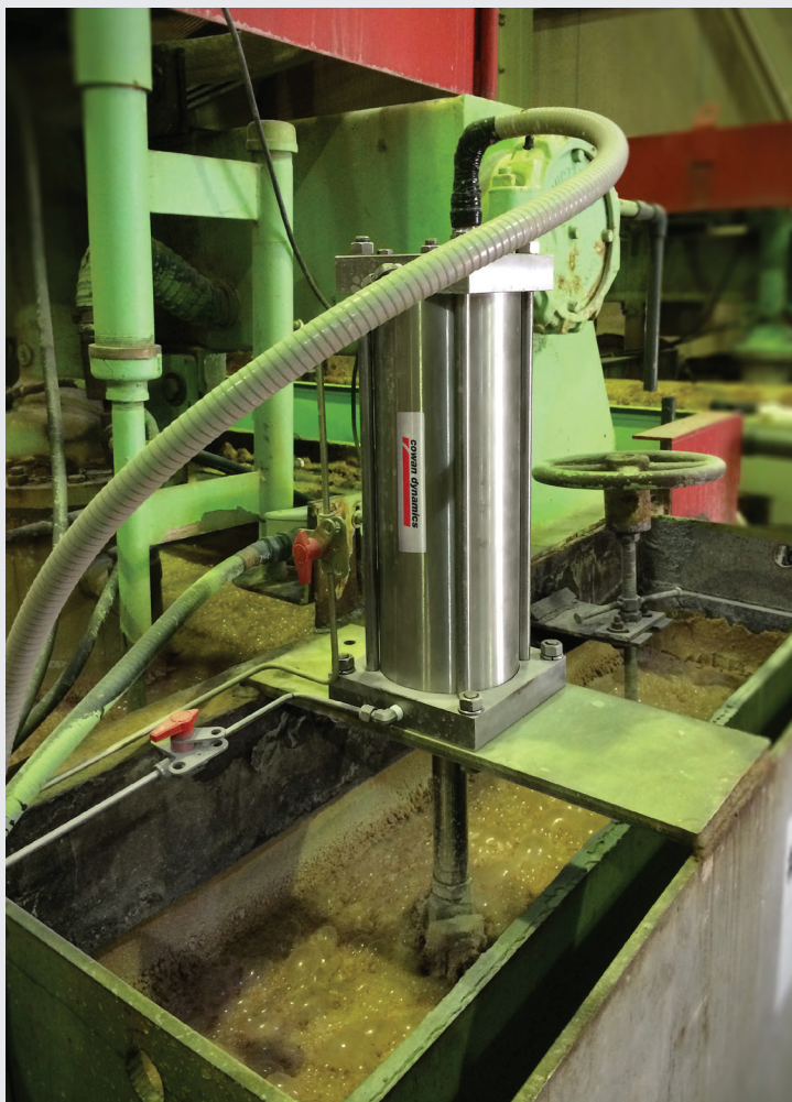
8" Bore Stainless Steel AT Series with remote positioner in a potash plant
